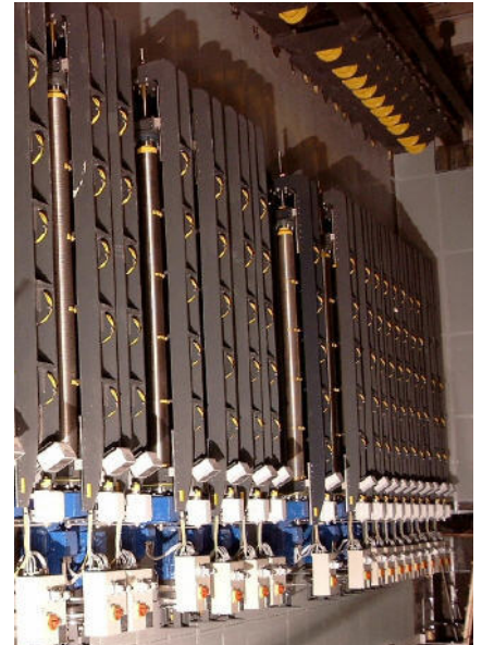
An installation of vertical spindle drives for flying bars – typical of an installation that must be well planned to allow future maintenance
